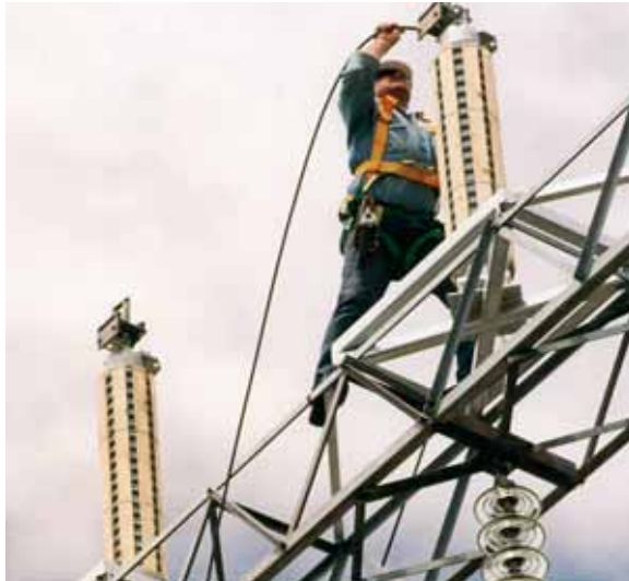
TRANSMISSION LINE COMPLIANCE: Post insulators were attached to a tower on the Tungatimah–Waddamana 110 kV transmission line by a crew from Aurora energy. The objective of the work was to raise the heights of conductors to meet contemporary conductor-to-ground clearances.
