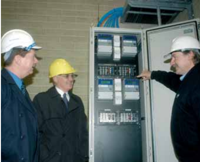
METERING: (from left) Shaun O'Loughlin, Aurora Energy, and Bob Neil, Department of Treasury and Finance, are shown NEM meters at Chapel Street Substation by John Peter, Transend.
