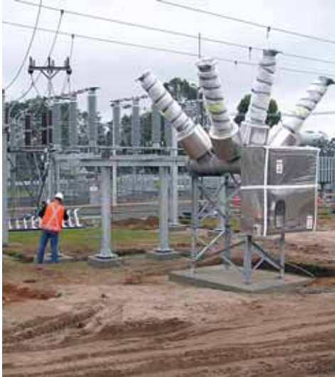
NORTH-EAST REDEVELOPMENT: A new 110 kV circuit breaker is being installed at Scottsdale Substation as part of the substation redevelopments in north-east Tasmania. (Photo courtesy of John Copas, Enerserve)
