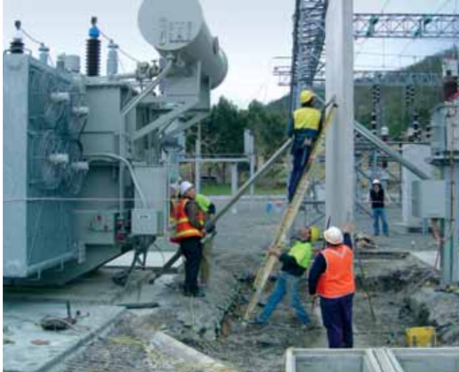
OIL CONTAINMENT: A blast wall was installed at Knights Road Substation, Huonville, as part of Transend's program to build contemporary oil containment facilities at all its substations.
