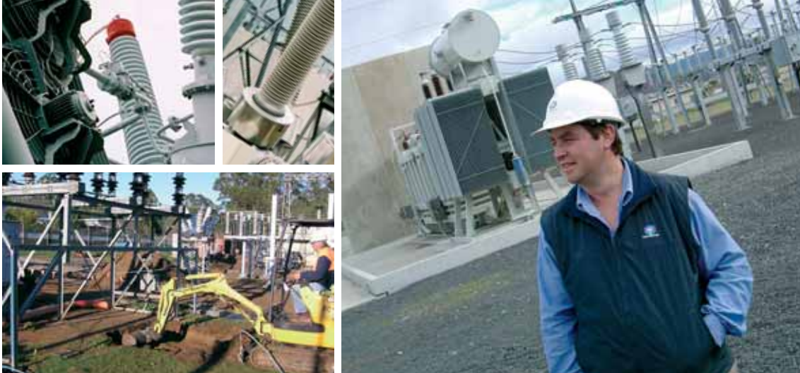
NORTH-EAST REDEVELOPMENT: Civil construction work at Scottsdale substation as part of the substation redevelopments in north-east Tasmania. (Photo courtesy of John Copas, Enerserve)
