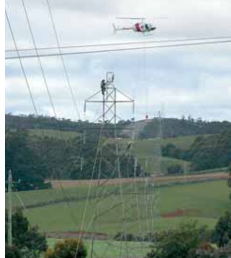
OPTICAL FIBRE GROUND WIRE An OPGW being installed on the transmission line between Burnie and Smithton substations. (Photo courtesy of Electrix Pty Ltd)
