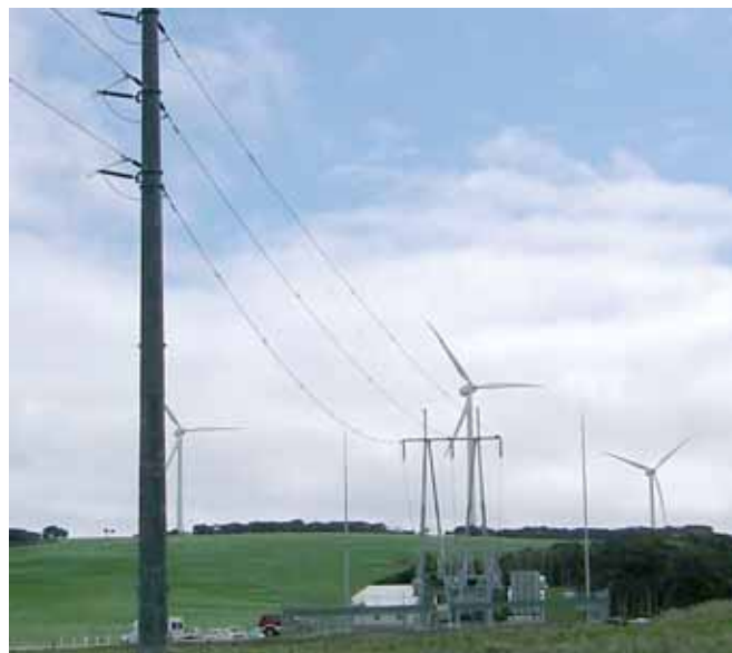
WIND FARM CONNECTION: Hydro Tasmania’s Woolnorth wind farm is connected to the transmission system by a new 110 kV line to Smithton Substation.
