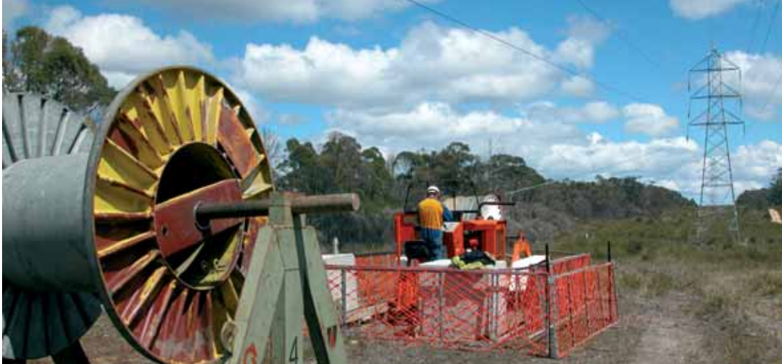
SECOND CIRCUIT: The second circuit being strung on the Burnie–Smithton transmission line as part of the redevelopment of the transmission system in the Circular Head area (Photo courtesy of Electrix Pty Ltd)
