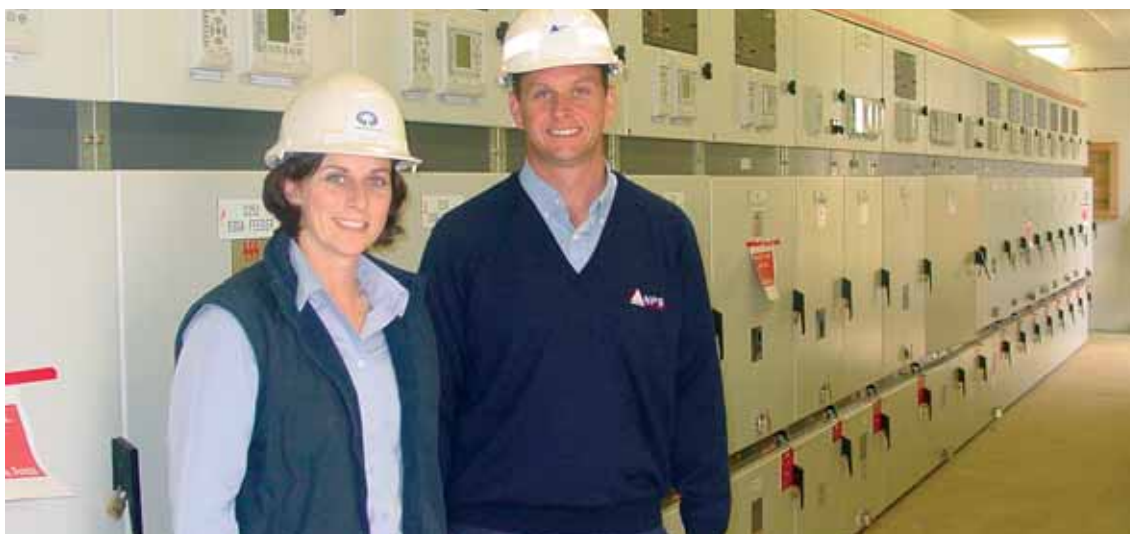
NEW SWITCHGEAR: Transend's Nicole Eastoe (left) and David Tossel, of National Power Services, in front of the new 22 kV switchgear at Burnie Substation
