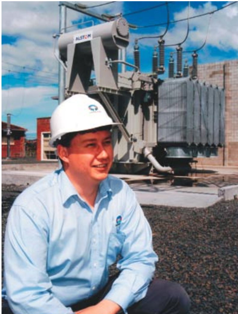
SUBSTATION REDEVELOPMENT: Adam King, Transend's Project Manager for the Creek Road Substation redevelopment, in front of one of the new transformers at the substation
