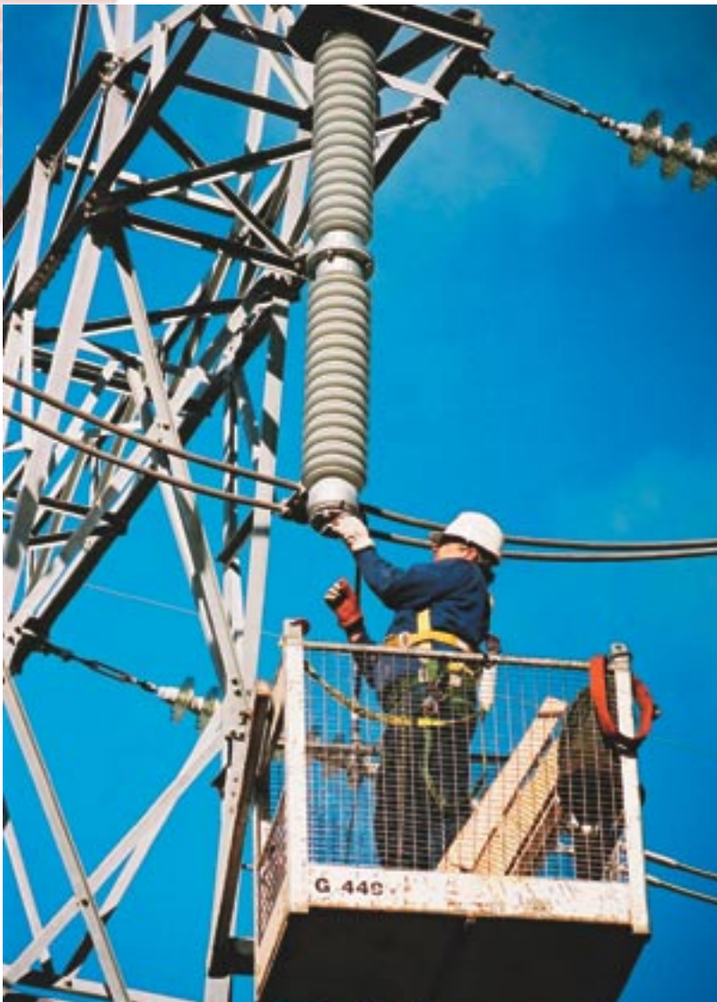
REPLACING EQUIPMENT: Phil Smith, who works for one of Transend's contractors, replacing post insulators on the 220 kV bus at Chapel Street Substation in Hobart as part of Transend's upgrade of the transmission system.
