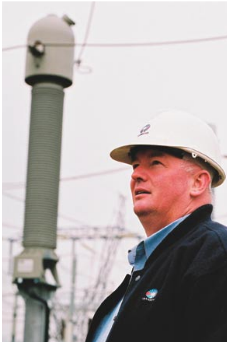
CHECKING ASSETS: Peter Smith, Senior Asset Officer – Substations, during an inspection of a substation. A 220 kV current transformer is in the background.
